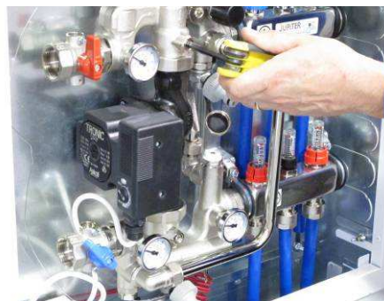
Close upper and lower integral pump isolating valves
