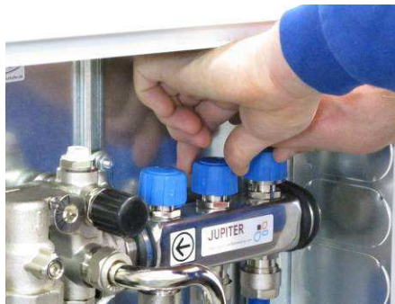
Once no more air bubbles emerge, simultaneously close the completed circuit and open the next one.
