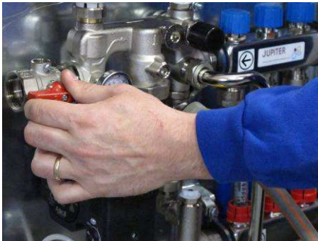
Close main flow and return isolating valves
