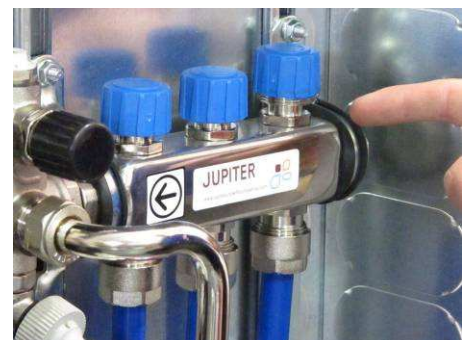
Screw down all blue caps on top valves except for circuit you wish to fill
