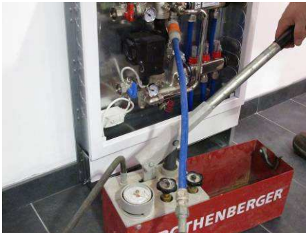
Once connected pump up to 8 bar. Once satisfied that there are no leaks, leave on test for a minimum of 1 hour. Once completed decrease pressure to 2 bar and then close return valve using cap. Release remaining pressure before removing test equipment from manifold. Remove hose and close cap. Re-open integral ball valves above and below pump.
