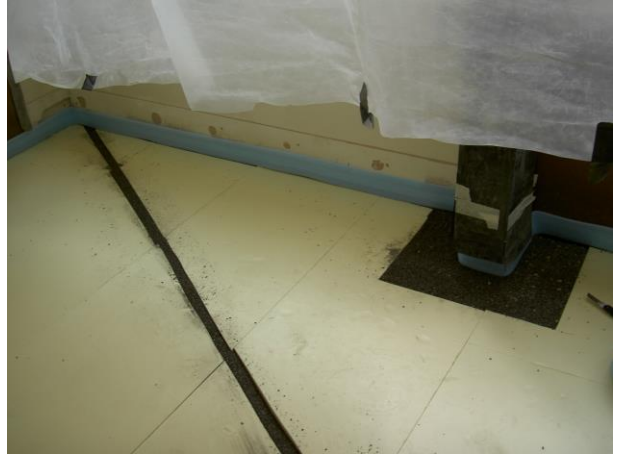
Channels left where insulation is installed up to conduits are filled with dehydrated slate ensuring channels remain full and stable
