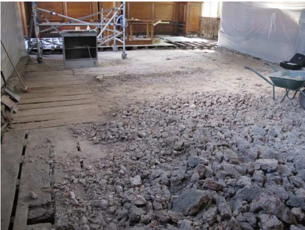
The existing floor was a combination of an old solid floor and old timber floors.
