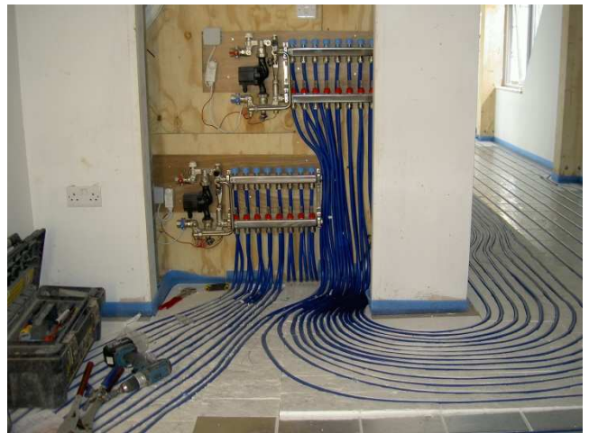
Space restrictions required that two manifolds be located in the same cupboard.
