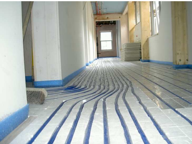
Shot showing flow and return pipework lying next to normal heating panels in long corridor.
