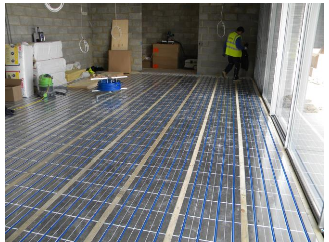
Leveldek system with installed underfloor heating
