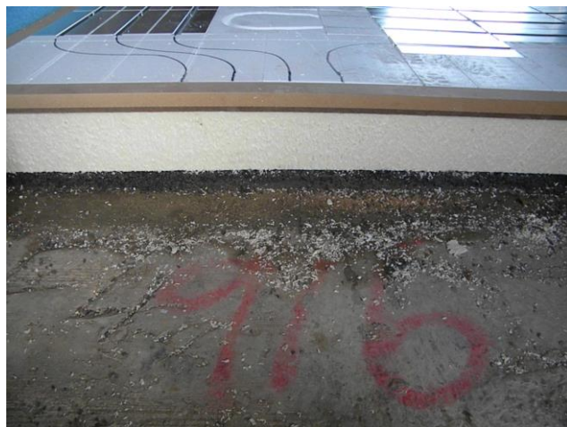
Floor construction made up of dry levelling, 500 kPa insulation, underfloor heating and SRT.
